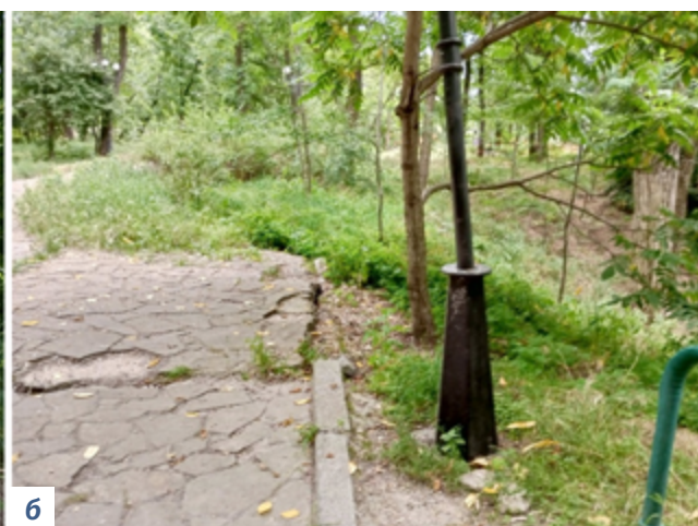
Fig. 2. Damage to the pavement and signs of a “drunken forest” near the St. Elijah Church (a); indications of suffusion processes on the slopes of Boldyna Hill next to the stairs (b). Photo by T.V. Kril, July 2025
