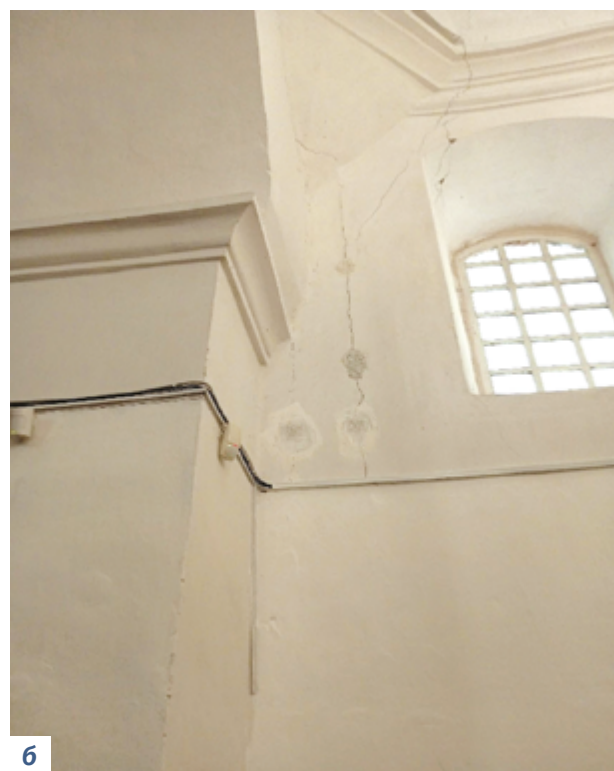
Fig. 8. Cracks on the interior walls of the St. Elijah Church with the 18th-century annex at the locations of deformation joints: north side (a), south side (b). Photo by T.V. Kril, July 2025
